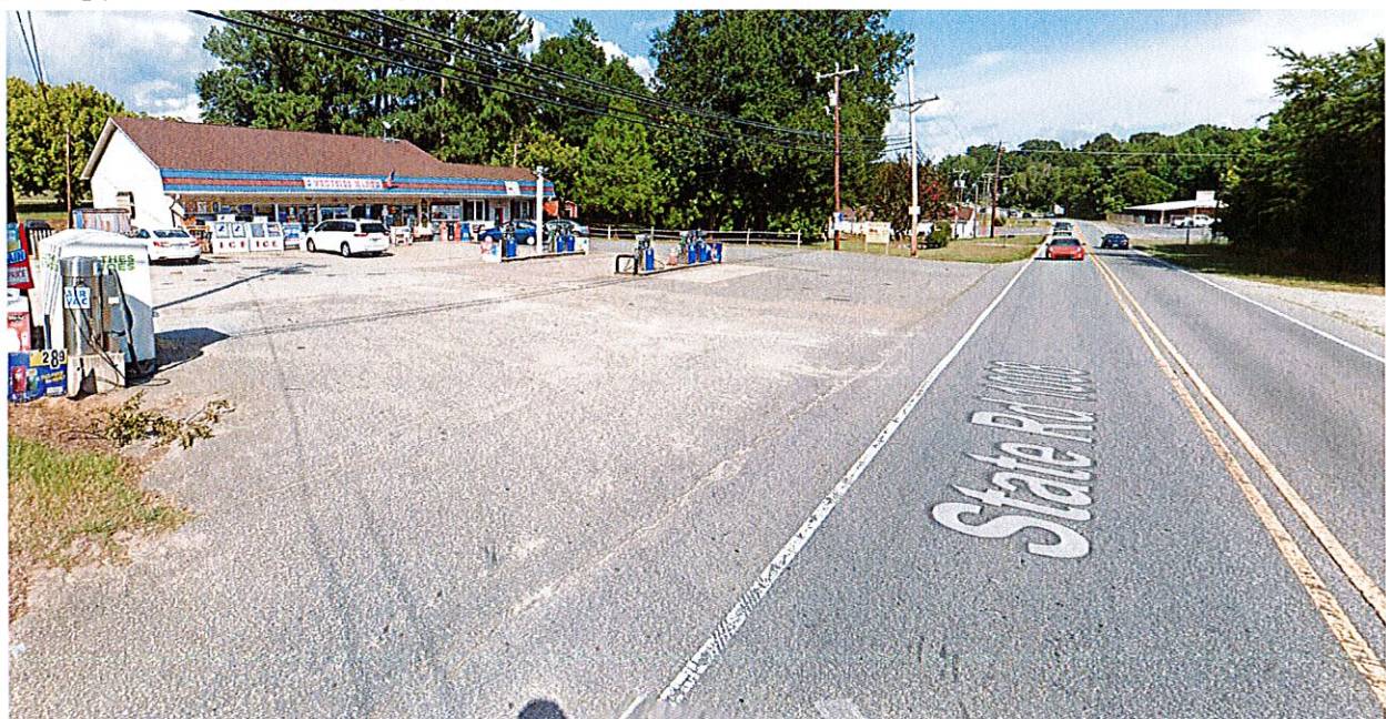
Canopy after Wind Damage 2021
