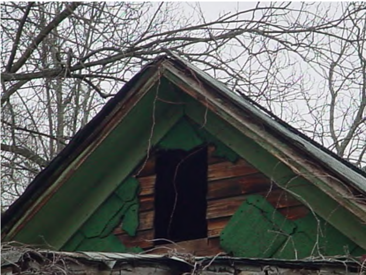
Gable vent missing
