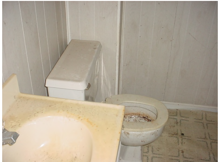
Bath fixtures, walls and floors unsanitary
