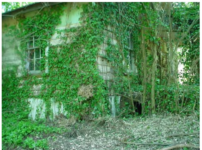
Grass weeds and vines overgrown
