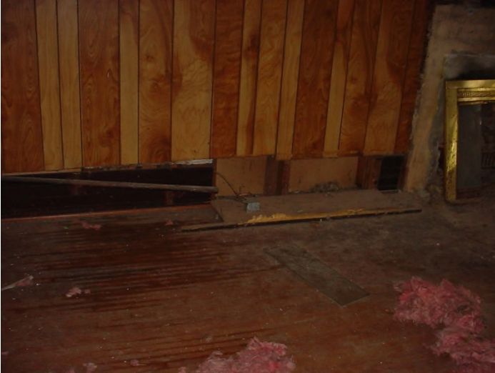
Holes at wall baseboards
