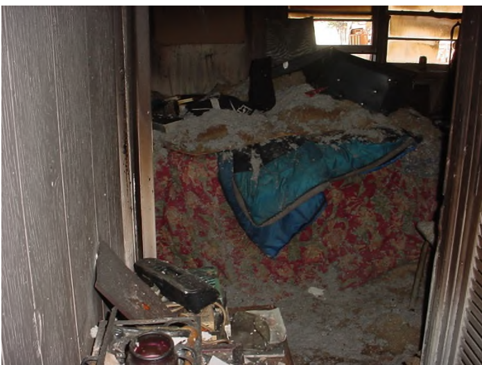
Ceiling insulation loose and fallen
