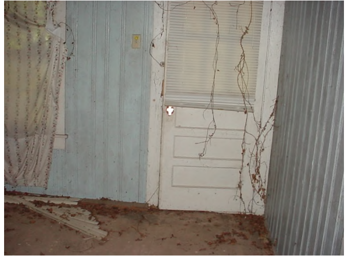
Door defective / Not weathertight Door hardware missing
