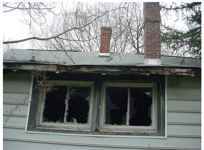
Fascia material deteriorated
