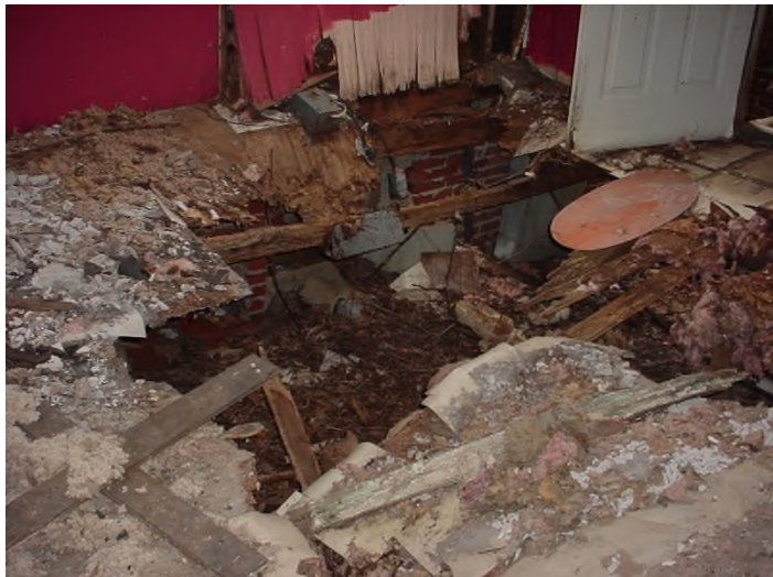
Holes in floors / joists deteriorated
