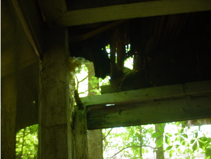
Holes in walls and ceilings
