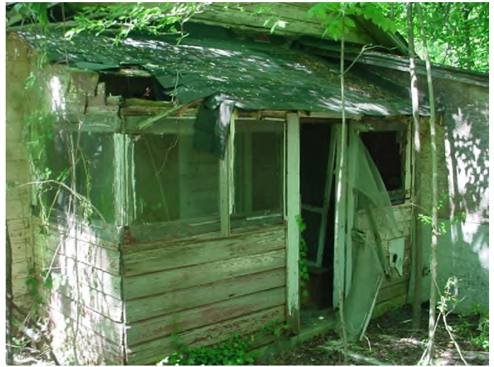
Holes in roof system / Door framing defective
