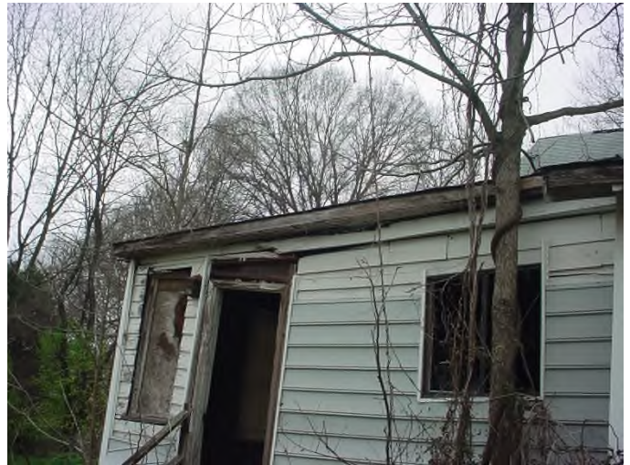
Windows broken / missing / not weathertight
