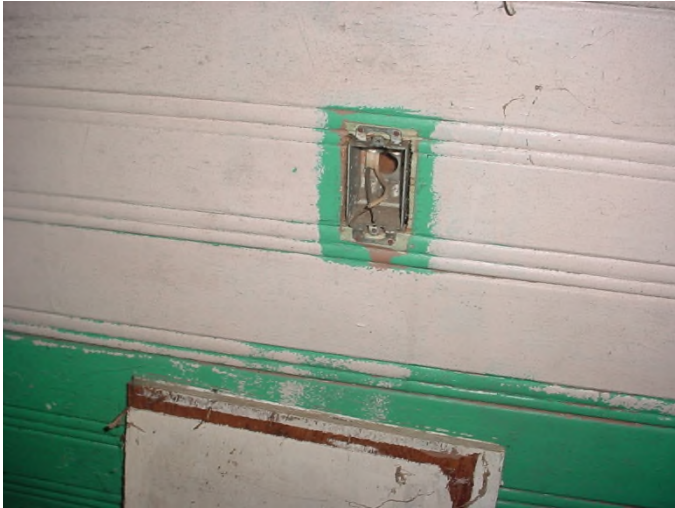
Electrical outlets missing / wiring exposed
