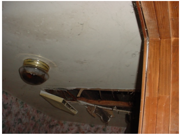
Holes in ceilings
