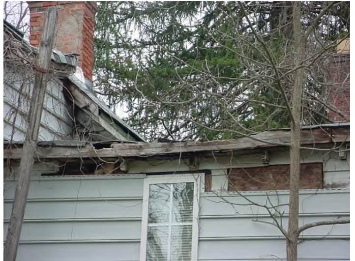
Holes in roof system / Fascia material deteriorated
