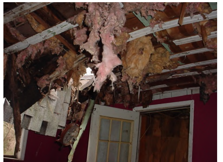
Holes in ceilings / insulation loose / hanging
