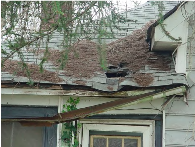
Holes in roof system / Gutters loose
