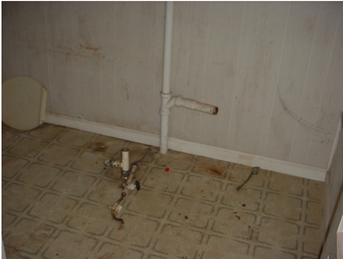
Bath plumbing fixtures missing
