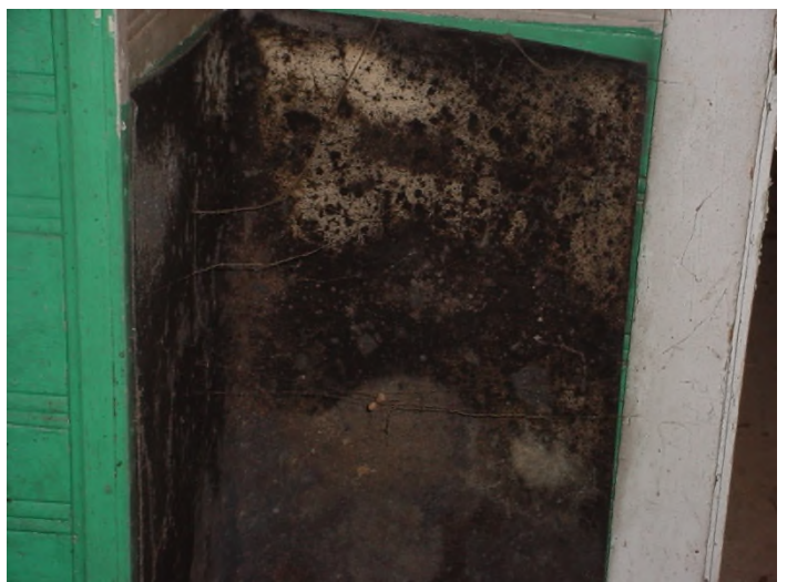
Mold / mildew at walls and ceilings
