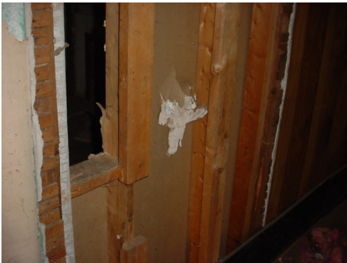
Wall studs exposed / Sheetrock missing
