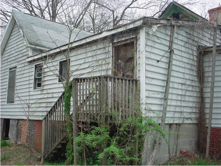
Hole in foundation wall
