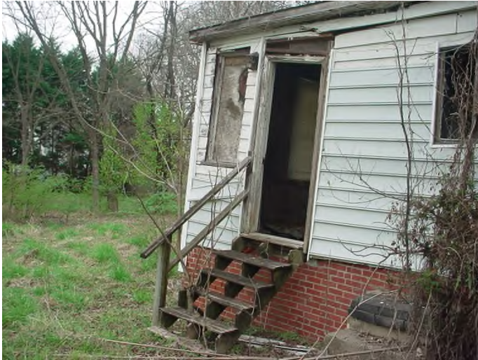
Rear steps defective / handrails missing
