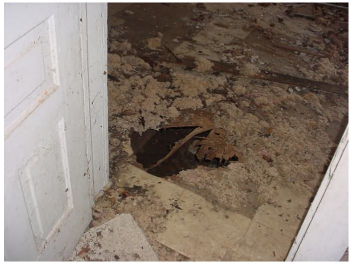
Holes in floors
