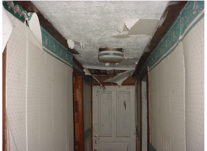
Ceiling material defective / Holes in ceilings
