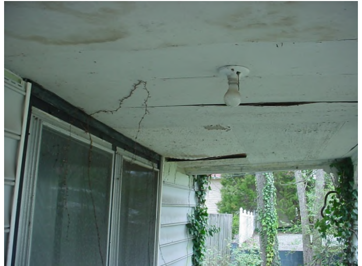
Porch ceiling water damaged / ceiling material loose / falling
