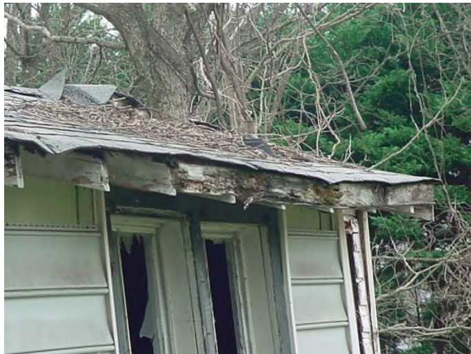
Rafter tails and fascia material deteriorated Windows broken / not weathertight
