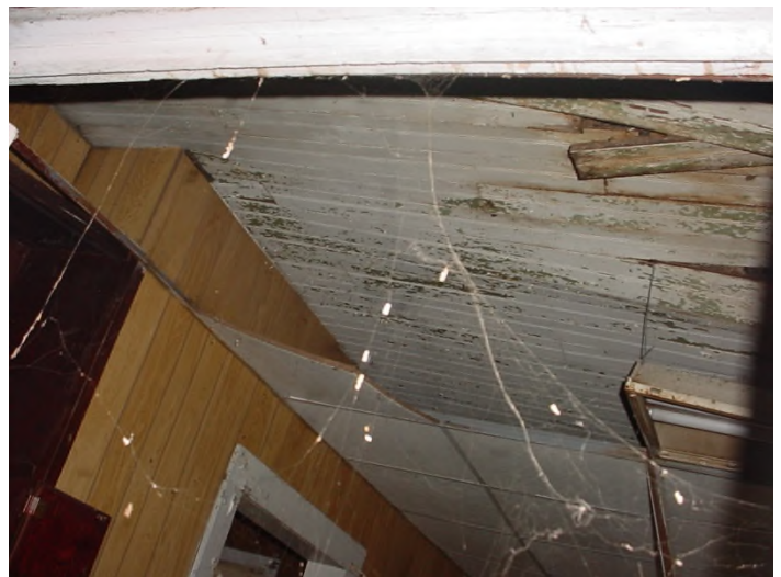
Ceiling material water damaged / loose / defective
