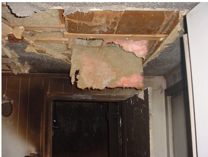
Insulation loose, hanging and water damaged
