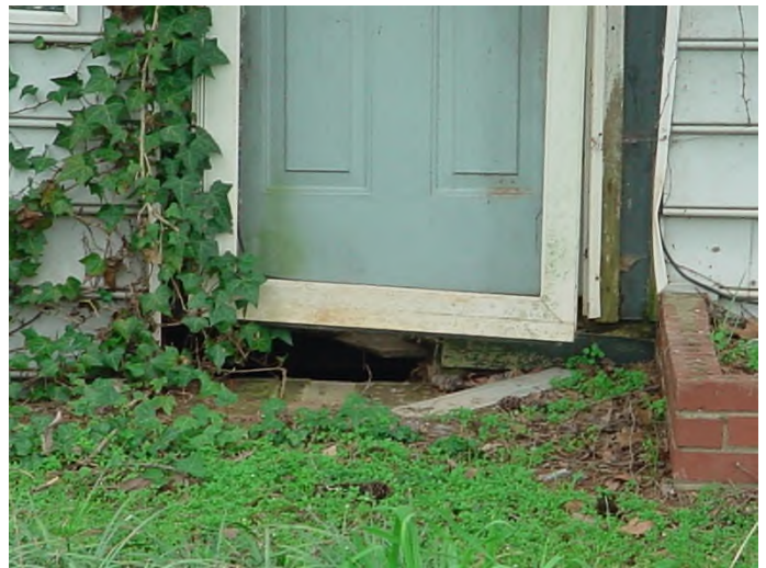
Sill rotted at entry door threshold
