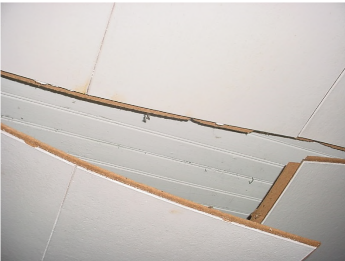
Ceiling material loose and hanging
