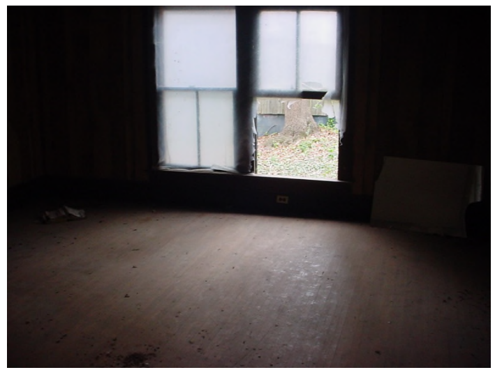
Windows broken / Not weathertight
