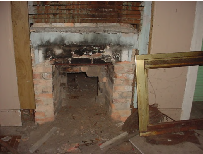
Fireplace defective / bricks loose / missing
