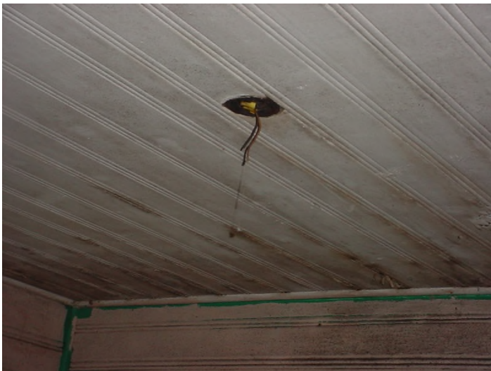
Ceiling light fixtures missing Electrical wiring exposed
