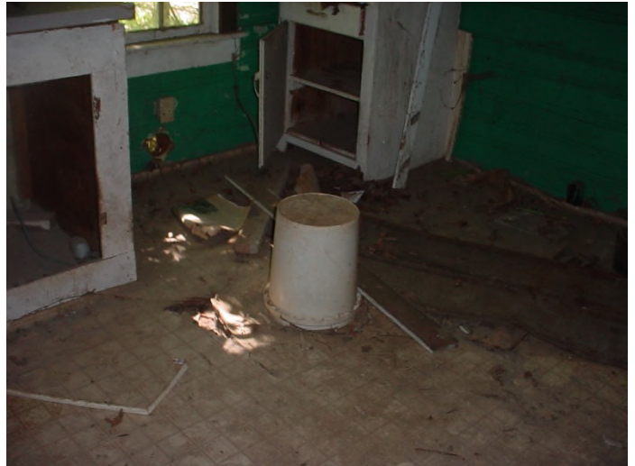
Cabinets defective (doors and drawers missing)
